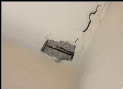
Spalling concrete at soffit slab
