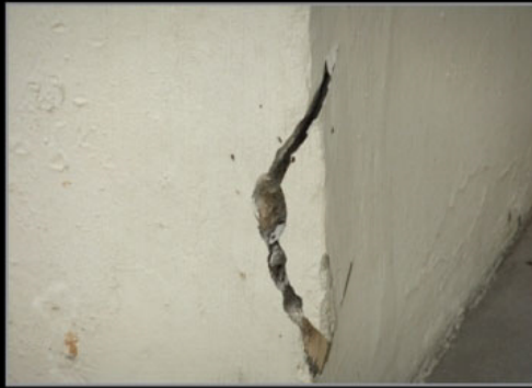
Crack found at column
