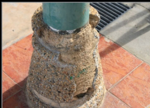
Debonded footing at linkway
